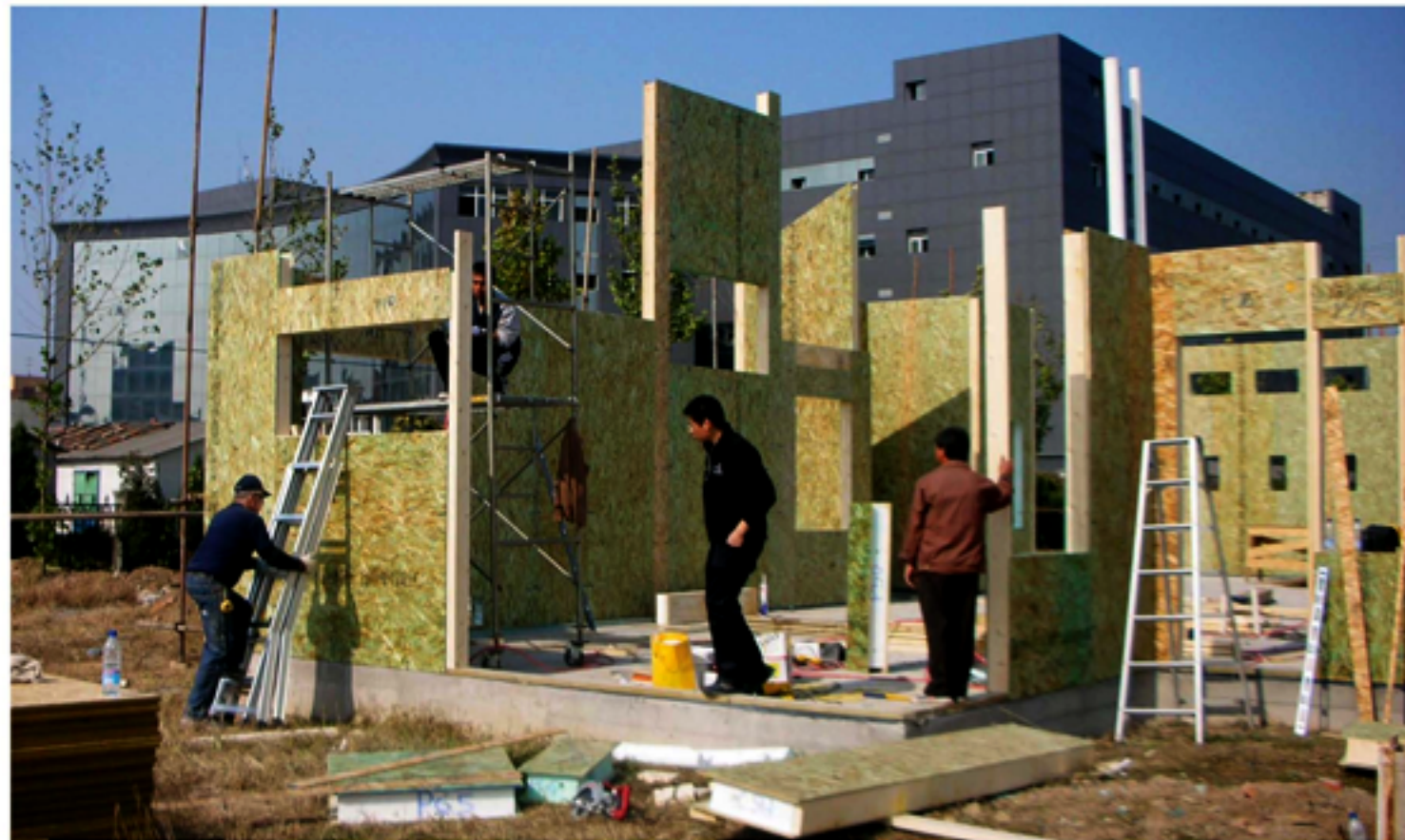
Local workers in Beijing, China, assemble Future House USA, made with panel sections designed and pre-constructed in Belgrade and Bozeman.
